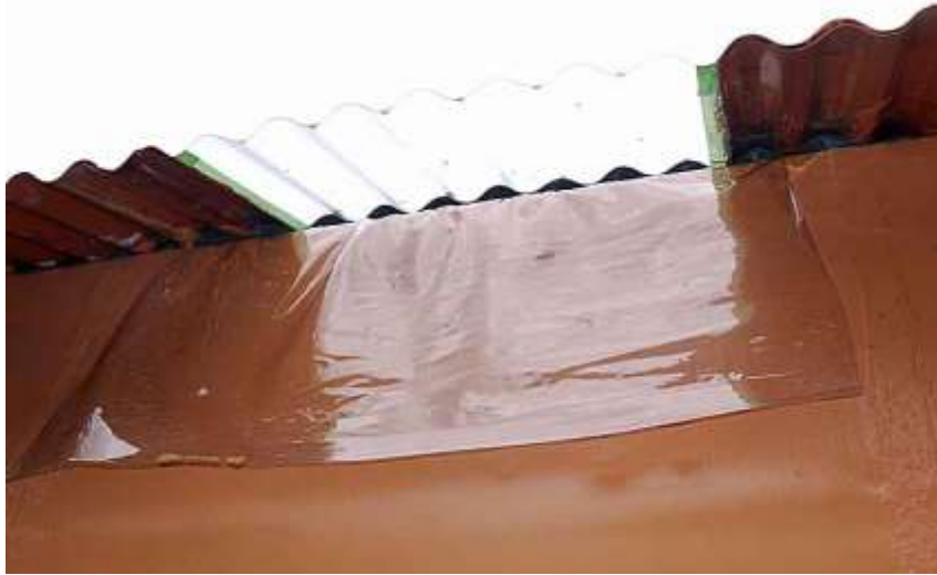
Skylight and PVU inner liner ready to roll up in the batten and fix outside
